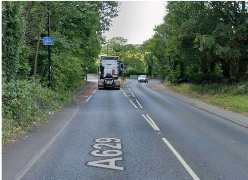
Approximately 100m of Worn Shared Use Cycle Lane on Cowley Hill - Google
